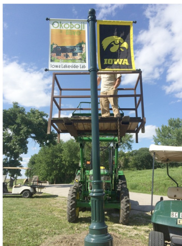
Matt Fairchild hangs the banners on one of the new poles along the bike path.
